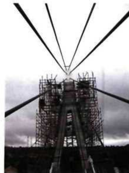
The pylon which supported the bridge had to be a very robust structure.
