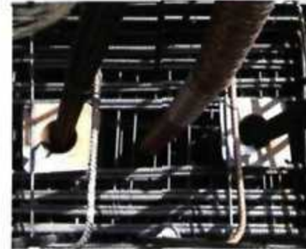
The combination of internal stressing ducts, reinforcing and attachments for cables resulted in an intensely congested space.
